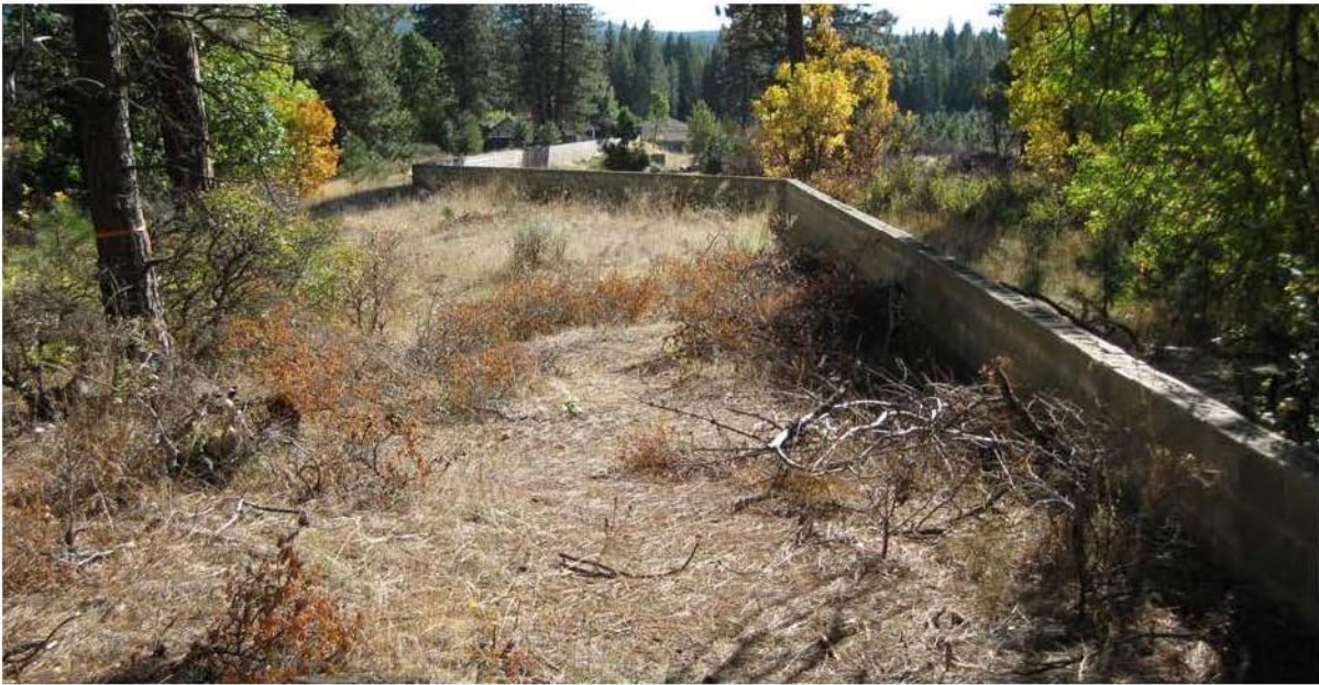
Burney Creek Floodwall
